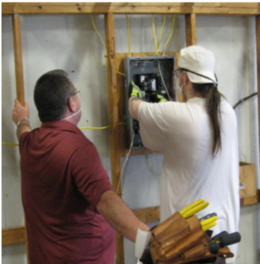
Electricity Instructor John Chapman oversees a student working on an electric panel.
